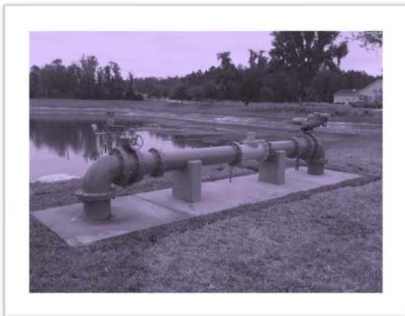
Southern Hills Plantation reuse storage pond 8AA, showing the delivery system piping from the City's Water Reclamation Facility.
